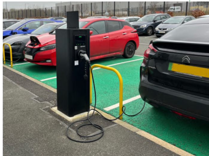
Electric vehicle charging points were installed at UK sites.
